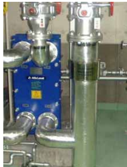
Outlet of hot and chilled water pipe in heart exchanger PT- 150DS
