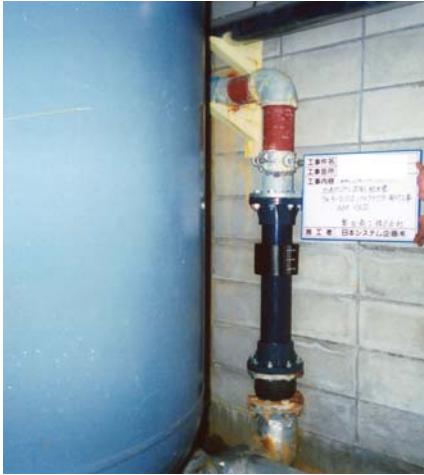
On outlet pipe of pressure pump
