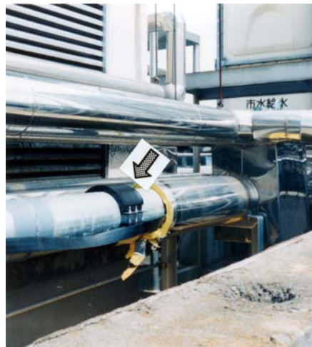
On outlet pipe of elevated tank PT-150DS
