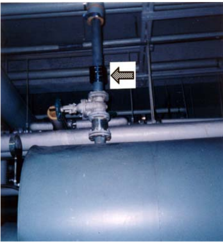
Storage tank PT- 75DS
