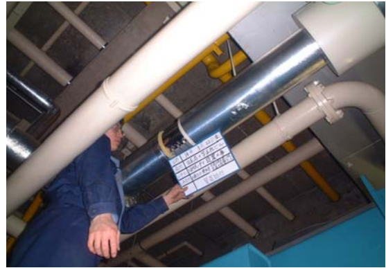
Outlet pipe from heating and cooling generator (PT-125DSx1)
