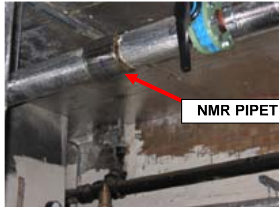
Outlet pipes of the hot water tank
